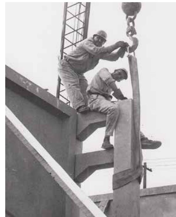
Local 361 members set precast columns and wall panels during construction of a Bankers Trust building on Rockaway Parkway and Avenue L in Brooklyn in June 1960.
