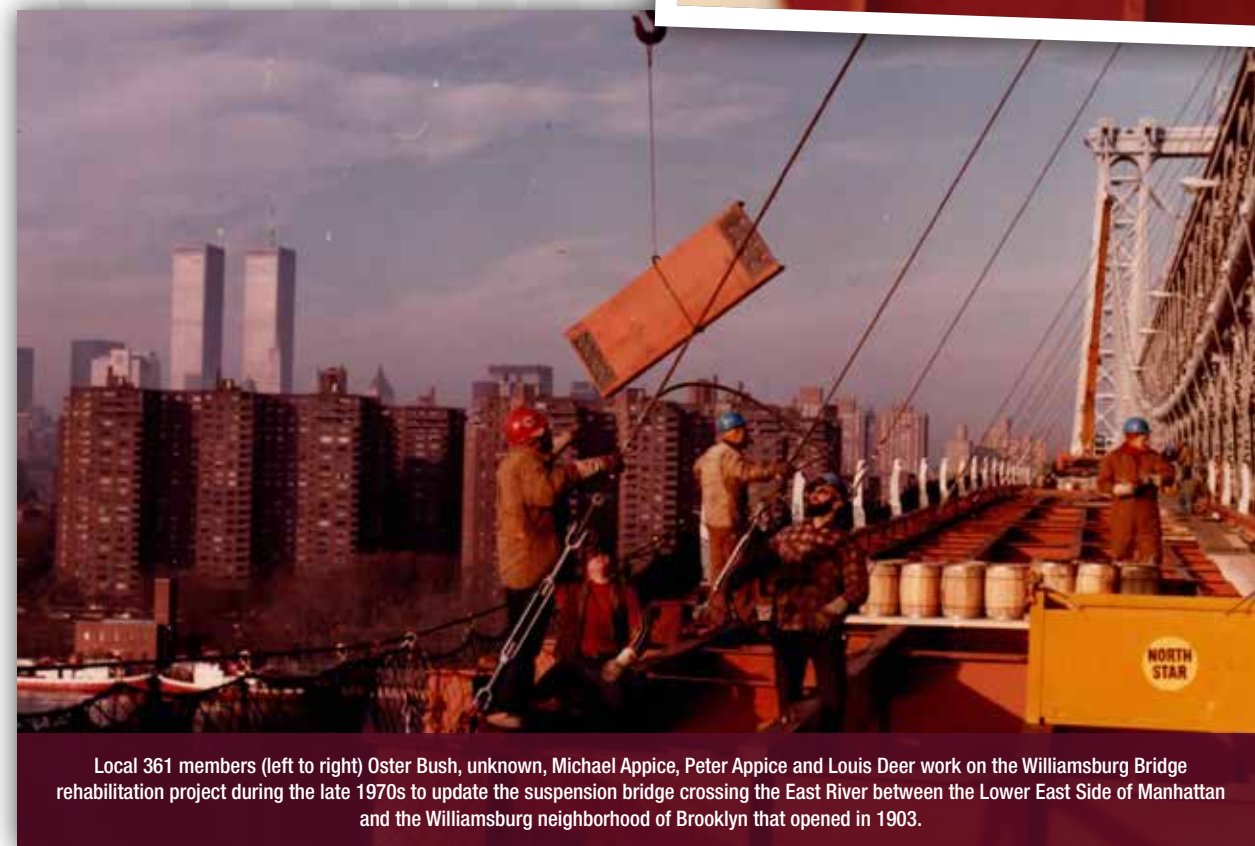
Local 361 members work on the new roadway steel for the Williamsburg Bridge rehabilitation project during the late 1970s.
