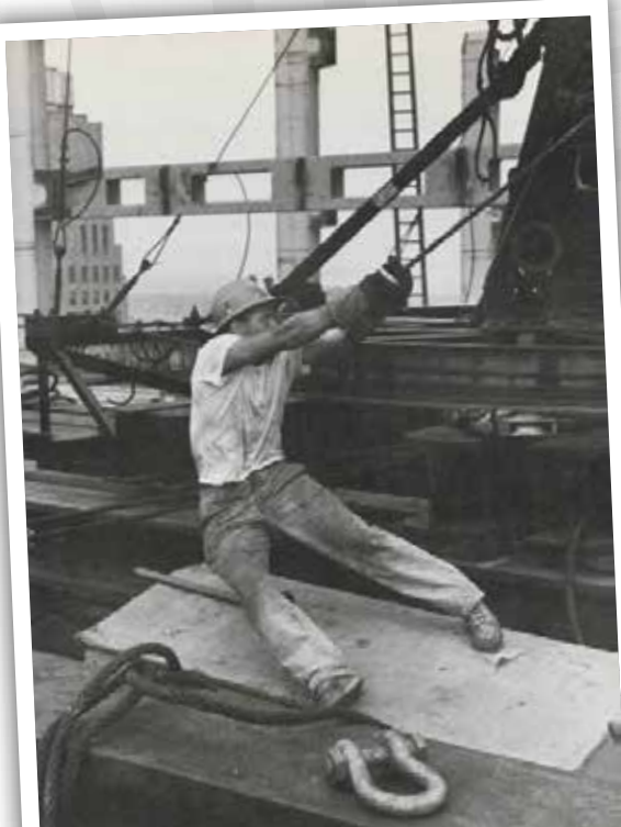
Local 361 Brother Richard Peddle II works on the tagline during construction of the Verrazano-Narrows Bridge in the 1960s.
